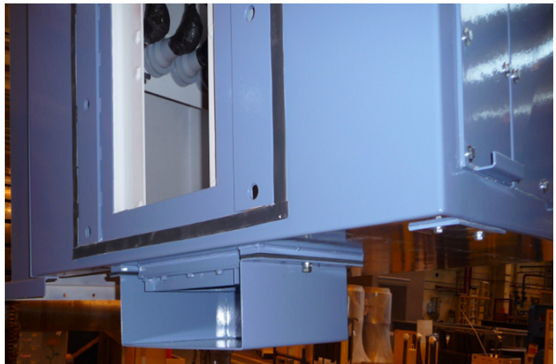
Exclusion vent shown installed on main terminal box.
